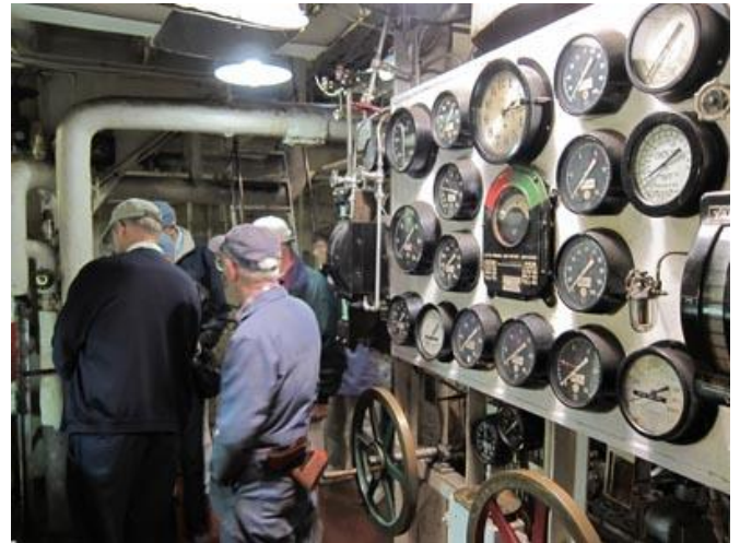
Engine Room Control Panel
